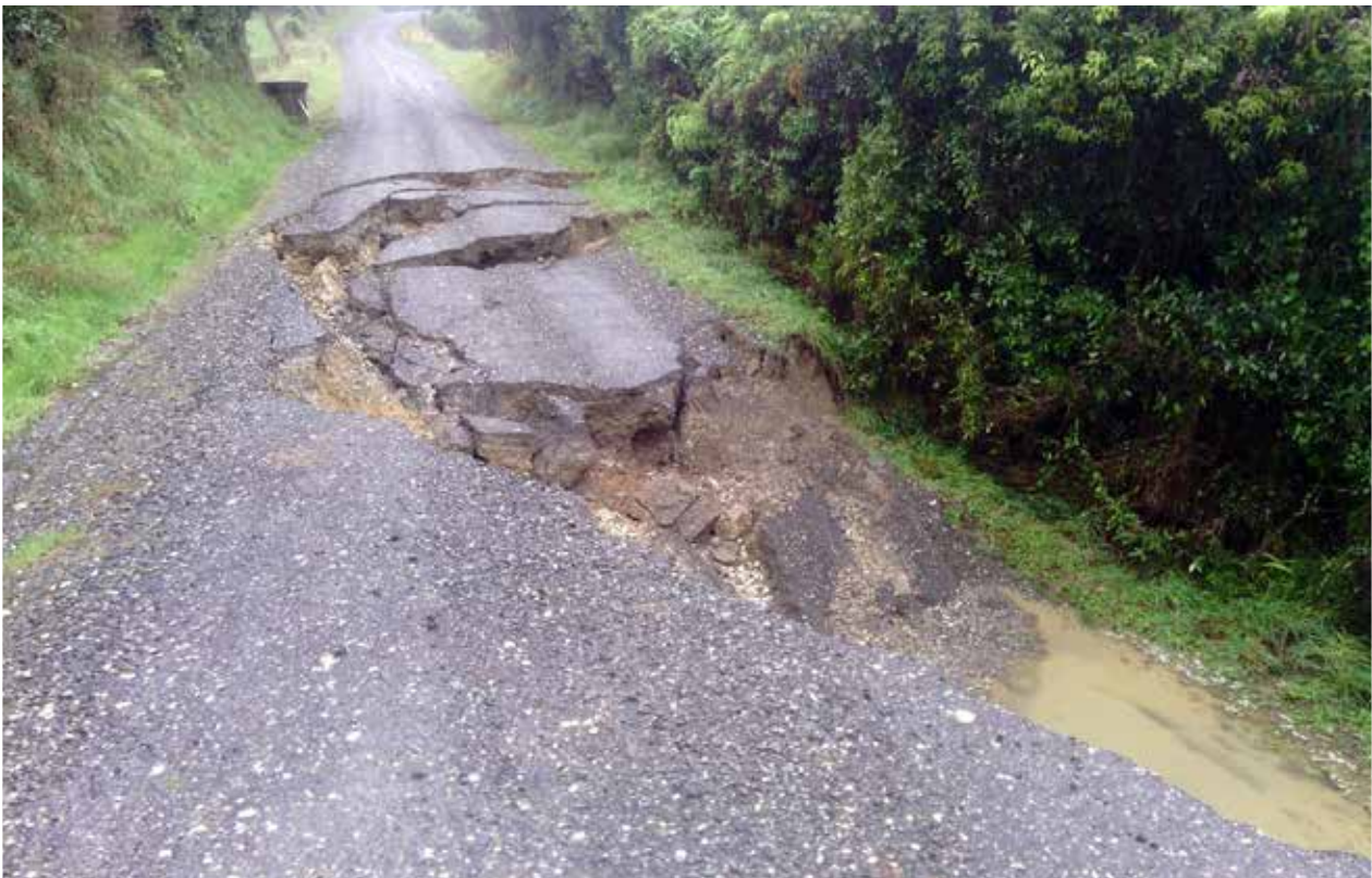
STORM DAMAGE TO PAEKAKA ROAD, PIOPIO - 5 APRIL 2017.
