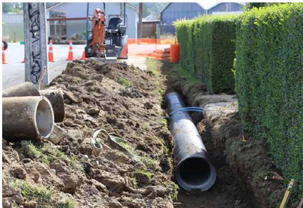
REPLACEMENT OF THE THE OLD STORM WATER PIPE ON EDWARD STREET WITH A LARGER DIAMETER PIPE - IMPROVING COLLECTION AND DISPOSAL OF STORM WATER RUN-OFF.
